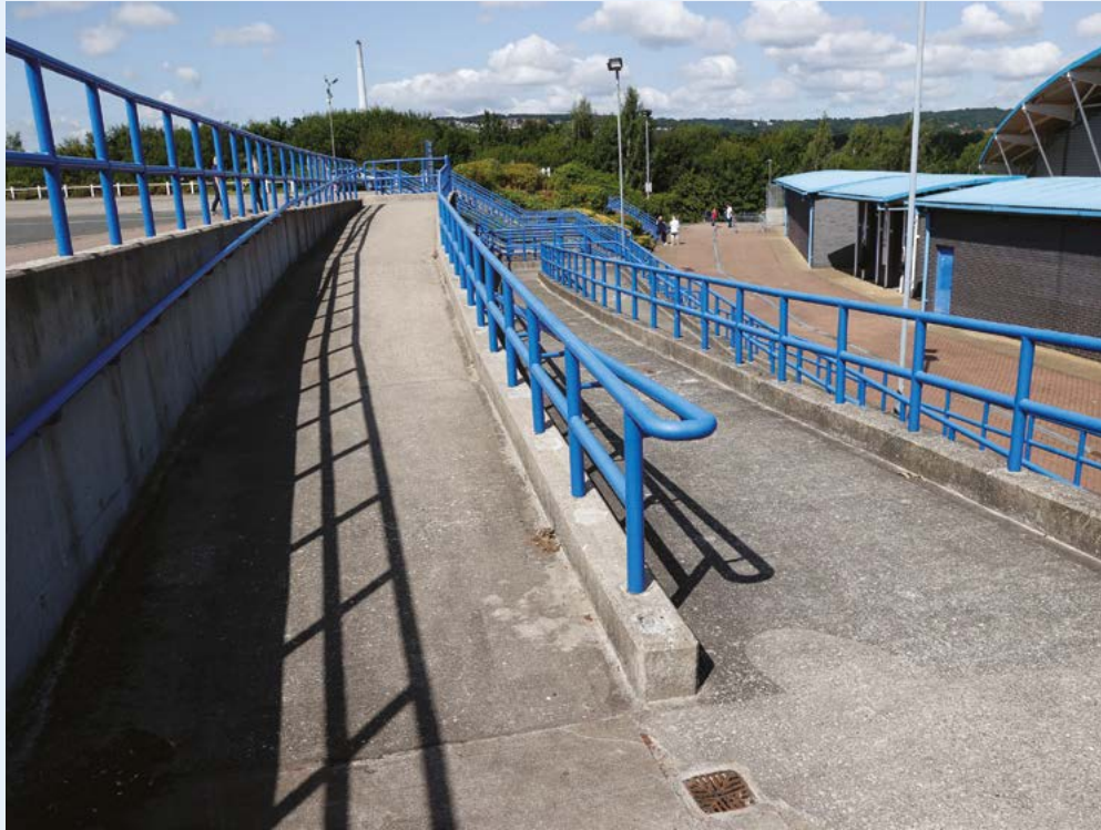
Figure 17 Ramp leading from St Andrew's Upper Level car park to the Magic Rock Stand
